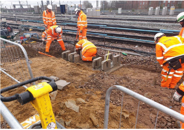
Civil gangs digging in PCC bases for location cabinets CD925 A, B & C
