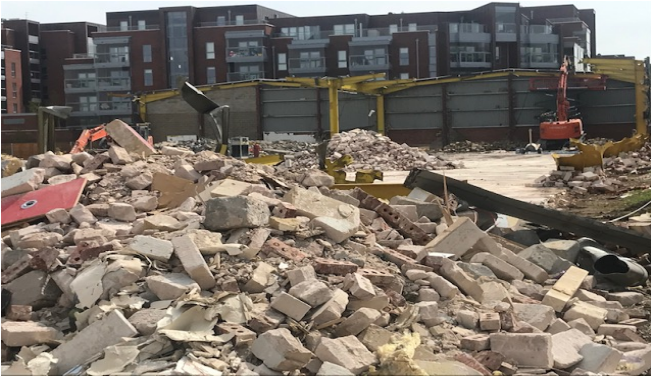
Demolition of Selco building commenced on 2 nd of April and is now complete
